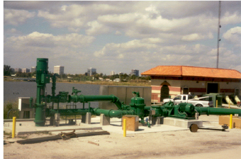
West Palm Beach, Florida ASR Well – 8 MGD Capacity Largest ASR Well in the World
